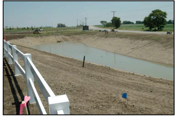
Whitetail cell awaiting MARS Aeration
